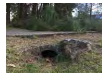
Turf swale with drainage under path
